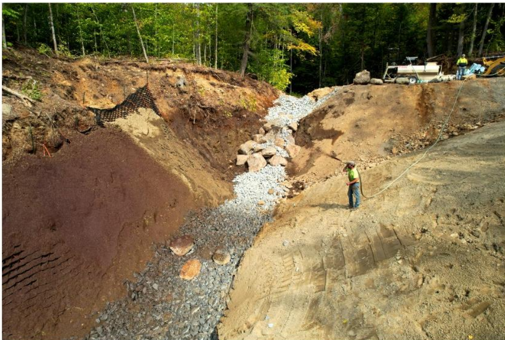
Technician Lenny Croote hydroseeds ProGanics Biotic Soil Media on top of GeoWeb to stabilize soil and prevent erosion.
