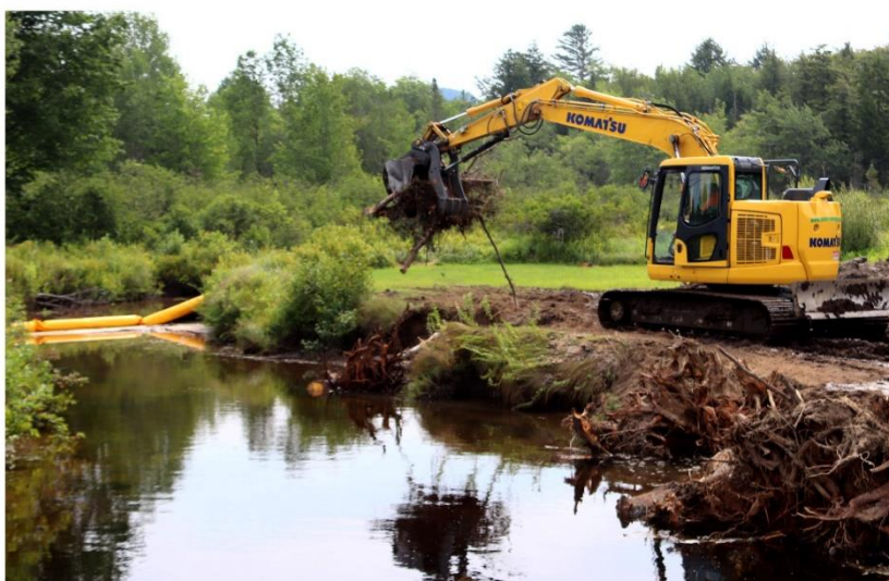
A heavy equipment operator installs root wad toe wood to create roughness and act as a barricade between water and streambank soils.
