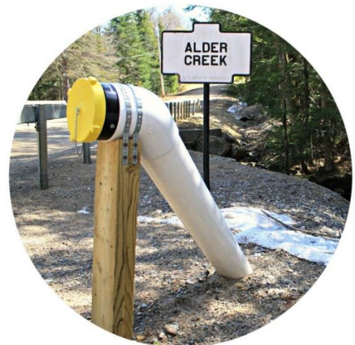
Dry hydrants protect public safety and aid fire departments.
