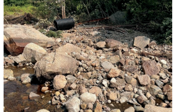
↑ On July 20, 2023, an 8-foot wave of water eroded and transported trees, culverts, and sediment downstream to the lower portion of Shaw Brook.
